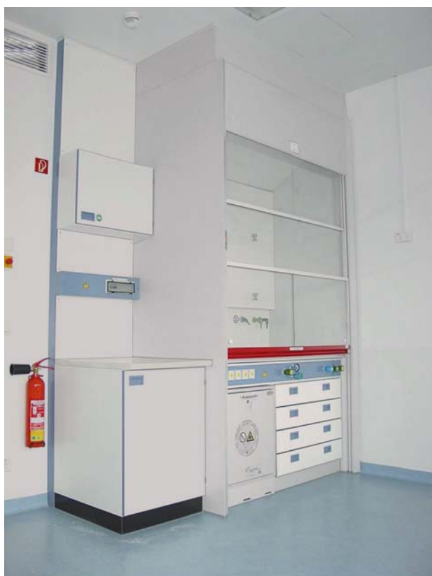
Photo: Fume cupboard with a fire resistant safety cabinet
